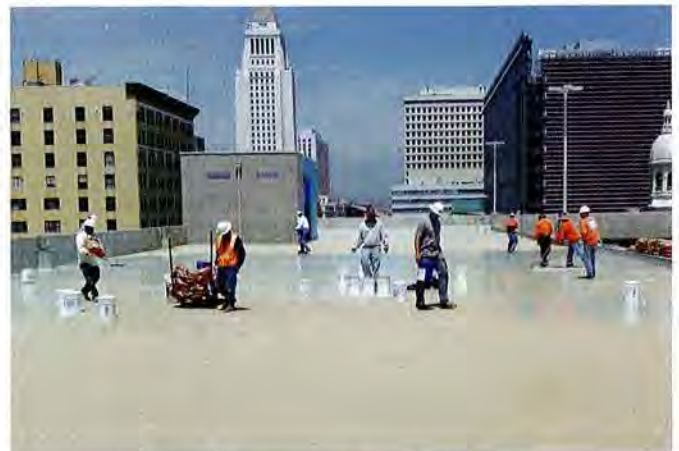
ABOVE ▲ The Pacific Waterproofing & Restoration, Inc. crew used squeegees to apply the Polyprime 21 primer to the substrate at a thickness of 5 mils (0.13mm) DFT. Following the pour, squeegee, and backroll application, the prime coat was allowed to cure for approximately six hours.
