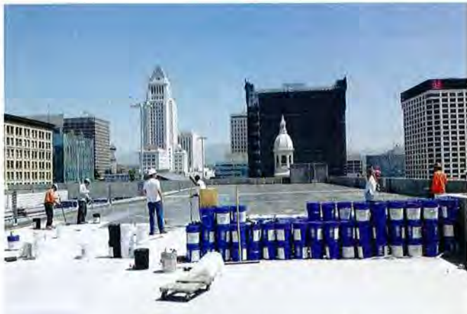
ABOVE ▲ The system specified for this high-profile project, Polycoat Products' Polyprime 21 and Poly-I-Gard 246SC are in compliance with South Coast Air Quality Management District (SCAQMD) strict low volatile organic compound (VOC) requirements.
