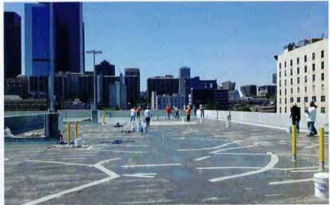
ABOVE ▲ Parsons explains, "Some of the cracks were 1/8" to 1/4" (0.32cm to 0.64cm) wide. Before any coating could be applied, the cracks needed to be repaired."
