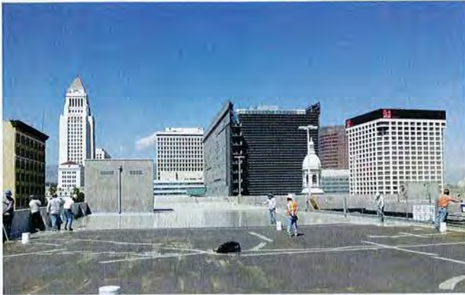
ABOVE ▲ Built in 2010, the 57,000 square feet (5,295.47m 2 ) concrete roof of the parking structure for the police headquarters for the City of Los Angeles Police Department sees a lot of traffic. Left uncoated, after a year of exposure and heavy use, it was in need of protection.
