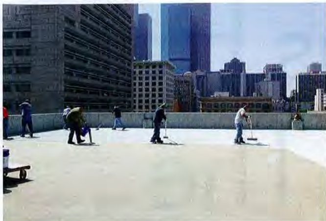
ABOVE ▲ An intermediate coat of Poly-I-Gard 246SC was squeegee-applied at a DFT of 11 mils (0.28mm). Following a sand broadcast, the topcoat was squeegeed, backrolled, and allowed to cure for 16 hours.
