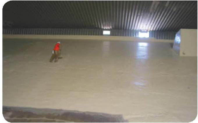
This 20-million-gallon (75,708,236 L) water basin covered 127,000 sq. ft. (11,799 m 2 ). And the project, which lasted three months, highlighted products that are NSF-approved to meet the needs of potable water — water that this crew has been drinking and will be drinking for years to come!
