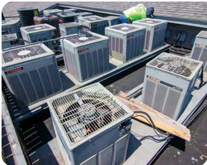
Each rooftop pit had 24 AC units and those had to remain operational throughout the entire summertime job. The crew had to work around the electrical lines and deal with their own heat concerns.
