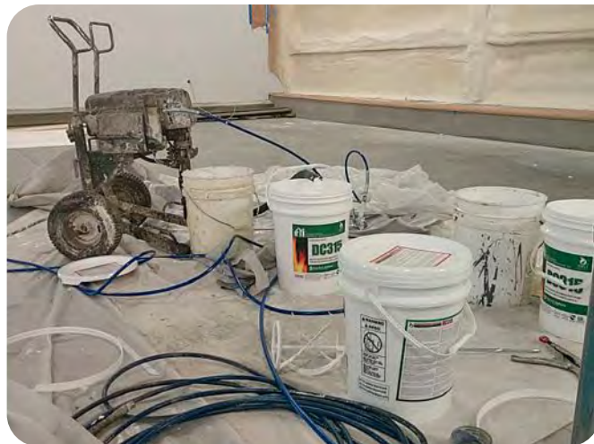
The coating systems varied. For the interior walls it included 5 inches of National Coatings' 2-pound SPF and 20 mils of International Fireproof Technology's DC315 Fireproof Paint.
