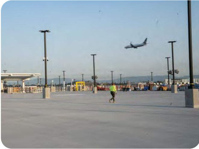
The concrete of the economy parking facility, which is owned by LAWA, was new, and it was broom finished.
